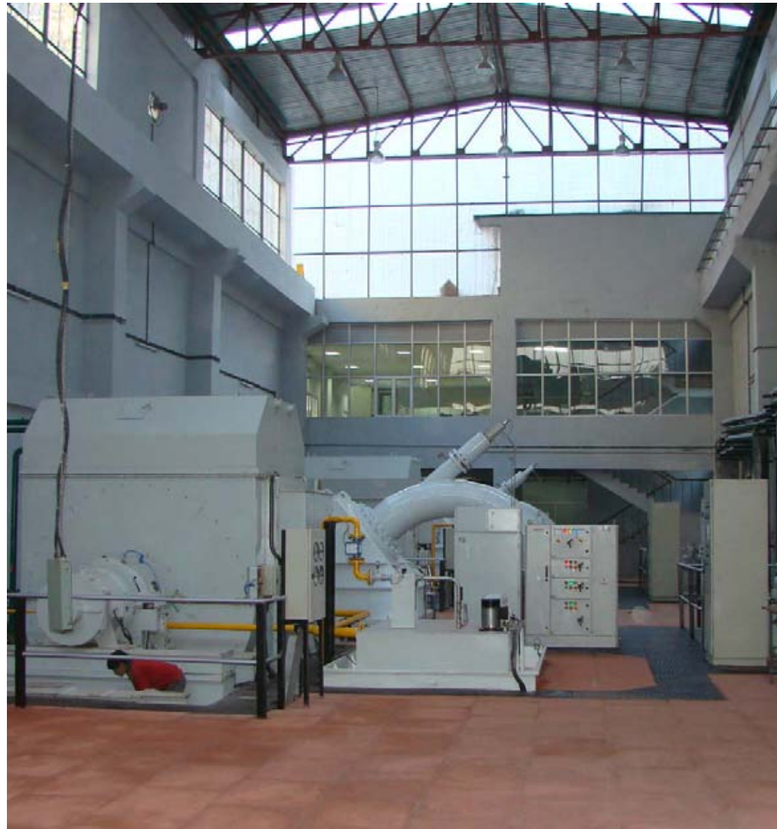
Patikari - 16MW Run-of-The-River Operational Hydro Power Plant
