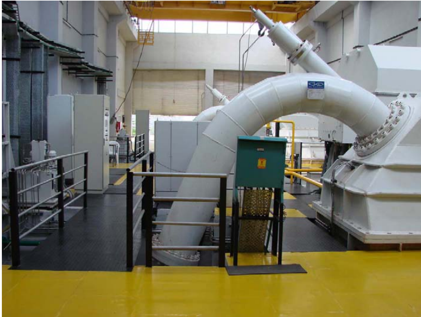
Patikari - 16MW Run-of-The-River Operational Hydro Power Plant
